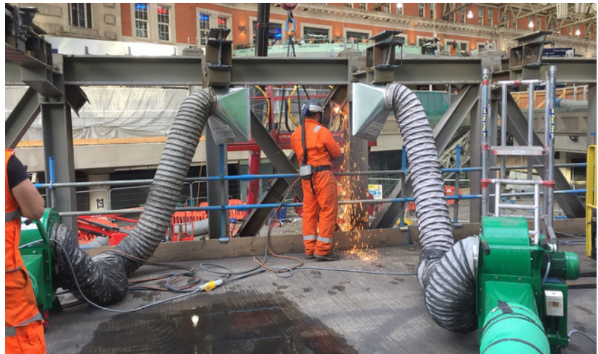
Fume extraction at London Waterloo Station during the £800 million Waterloo and South West upgrade
