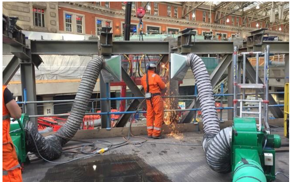
RVT's Ventex® 300m fans extracting hazardous fumes at a railway station
