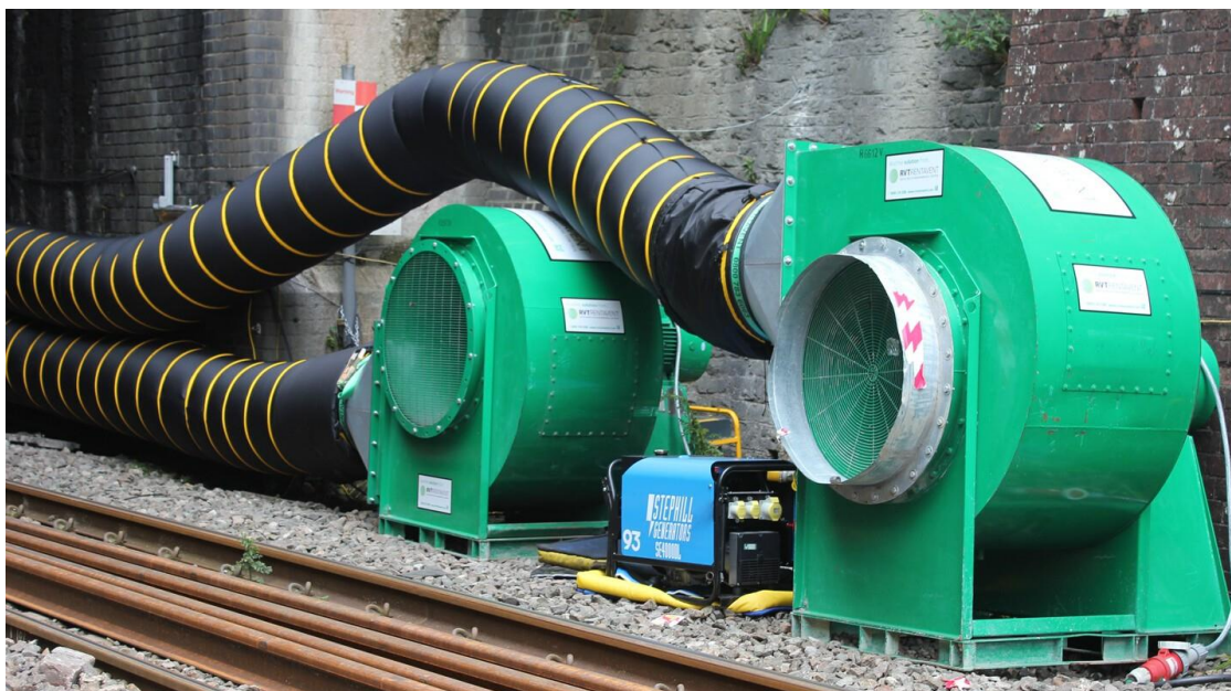
RVT's Ventex® 800CF centrifugal fans on site at a railway tunnel
