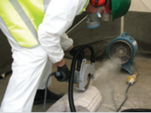
A localised system in use within an enclosed space.
